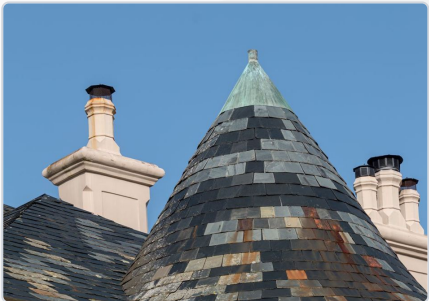
1c Rear stack from the ridge: flashing no longer sealed to the slates
