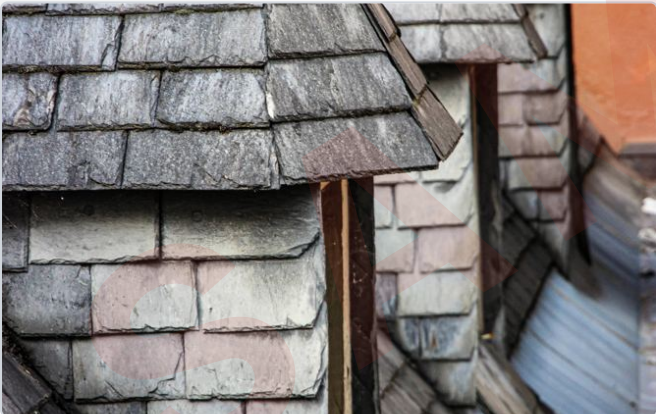
2a Front pitch: slipped slates and previous tingle repairs by the valley
