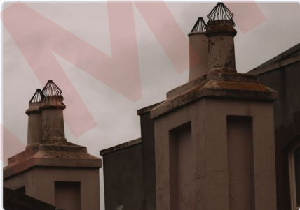
1b Rear stack: vegetation in the joints and lifted flashing at the base
