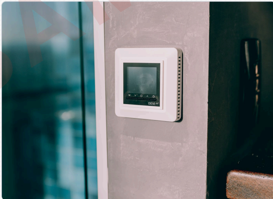
Room thermostat, hallway
