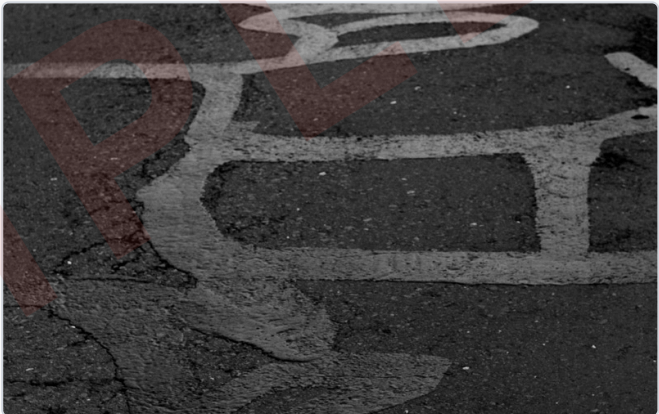
2b Bays: cracked and patched surface, markings faded but legible
