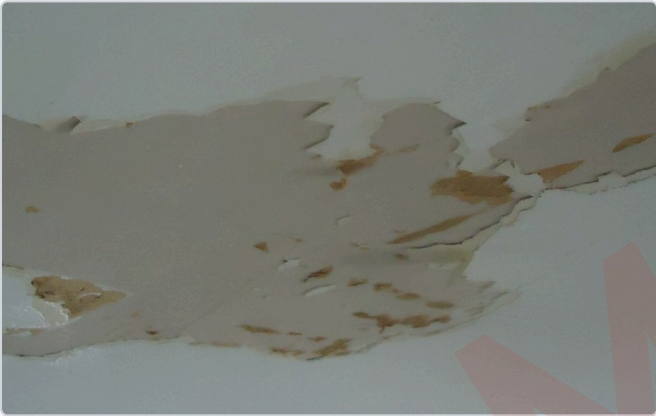
4a Tide-marked stain below the valley gutter; dry at the time of inspection
