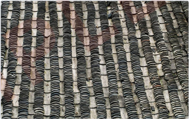
3b Ridge: weathered mortar and two moved tiles
