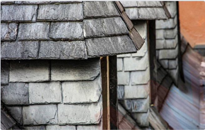
3a Front pitch: slipped slates and previous tingle repairs by the valley
