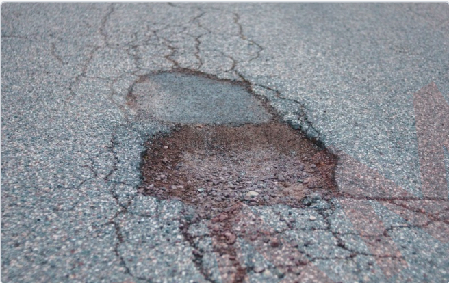
2a Entrance: larger pothole with crazed, loose surface around it
